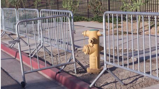
Swing gate allows access to fire hydrants
